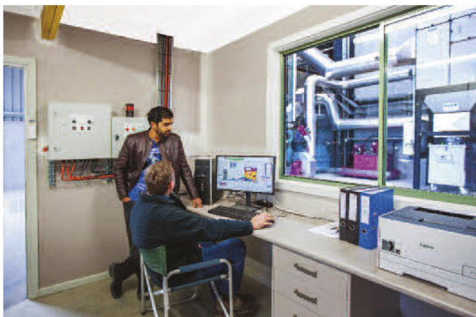
Control room for onsite and remote monitoring of the energy plant.
