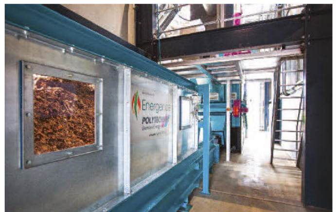
Cross conveyor pushing fuel from the bunker into the furnace.
