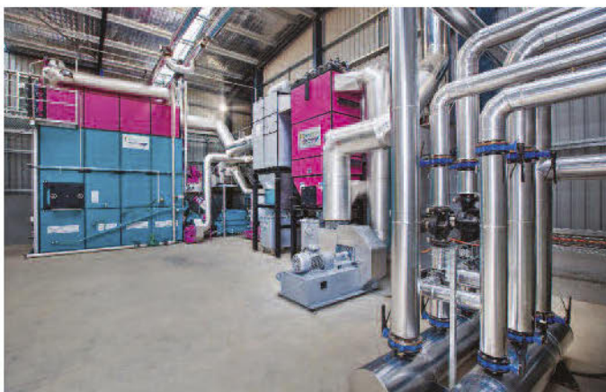
1.6MW heat plant showing (left to right) the furnace, muticyclone, air preheater, ID fan, pump unit.
