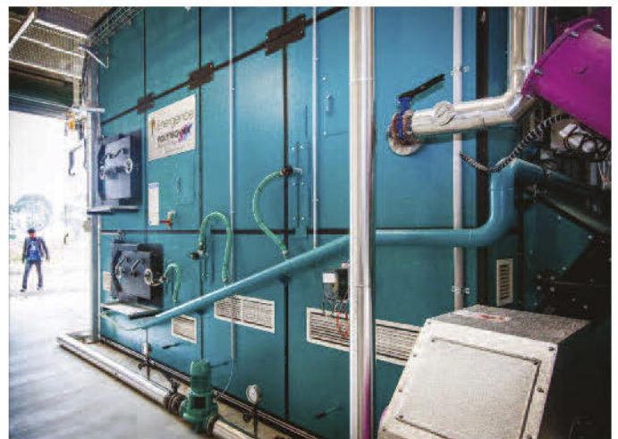
Furnace, inside of which combustion of biomass occurs on a reciprocating step grate.
